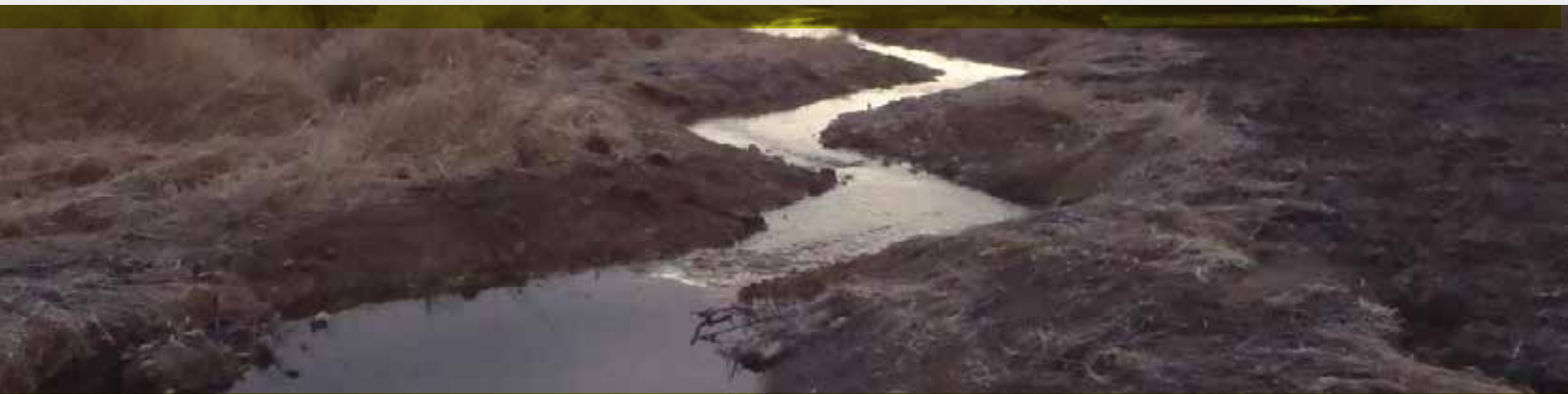
The completed Bauman Creek channel, awaiting erosion blankets and seeding with native plants. Photo by T. Woodcock
